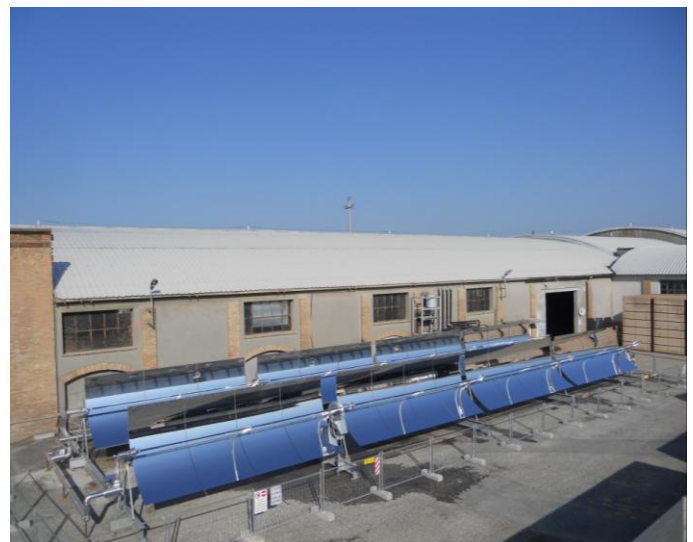
Solar parabolic collectors
